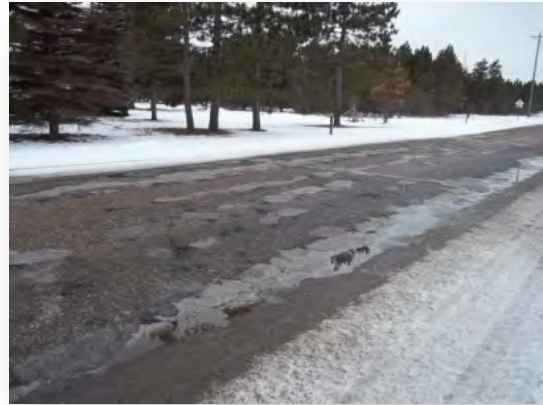
Figure 8 - Wilcox Bridge Road Pavement Conditions
