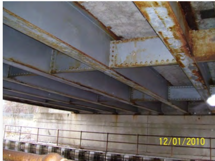
Figure 10 - North Down River Road Bridge corroded and undersized beams
